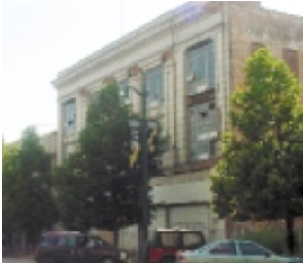
A number of serious challenges to preservation exist Downtown. The Schmidt's Garage property (top) and the Vernor Building (bottom) on the 700 Block of Main Street, for example, are contributing buildings to the historic district, but years of neglect make them vulnerable. Even so, planning continues to discover ways to preserve important elements of the structures as part of the 700 block renewal. (Source: The Urban Design Project)
