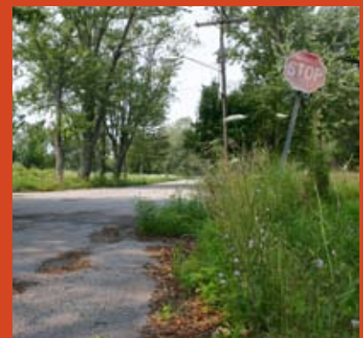
Overgrown streets and sidewalks at the corner of Wheatfield and 101st on the eastern side of Love Canal
